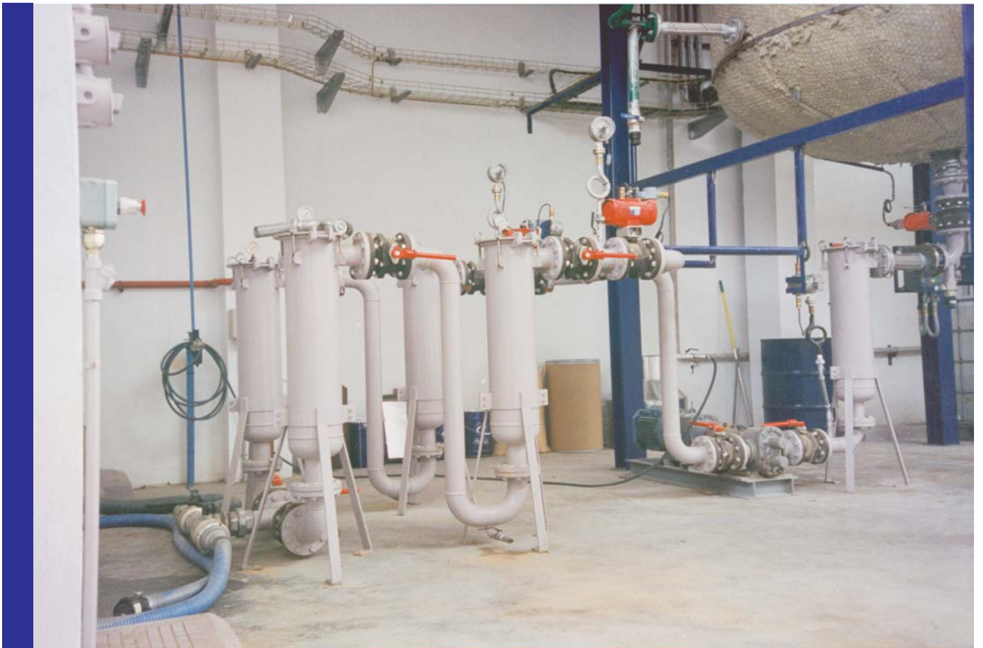
Automatic filtering equipment
