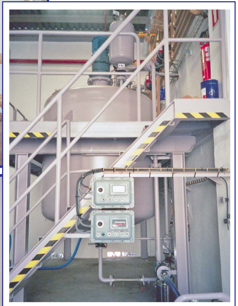
EExd control panels
