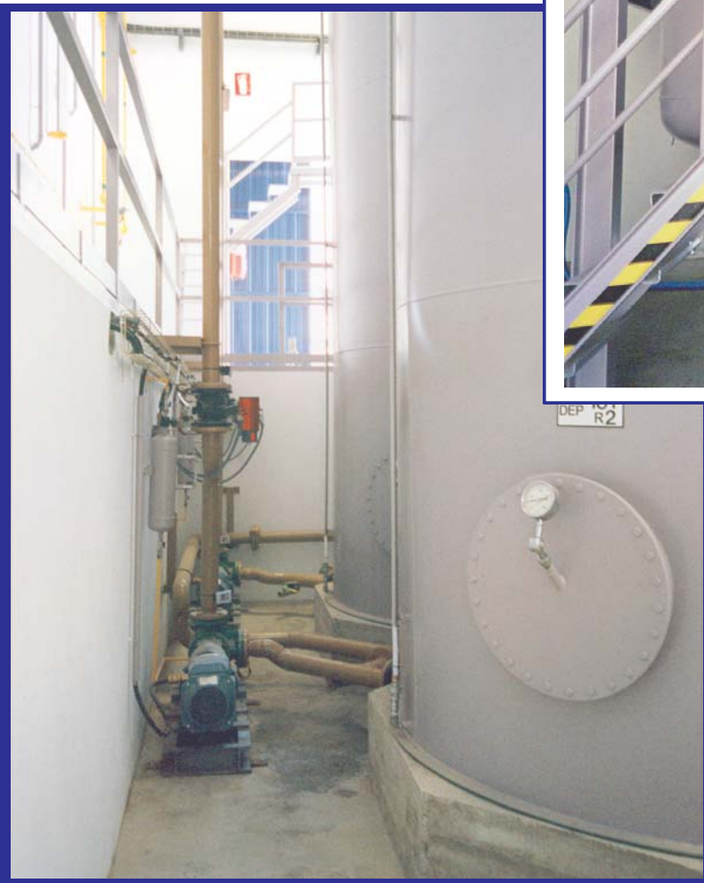
Isocyanates storing tanks
